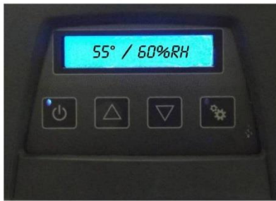
Local Interface Controller
